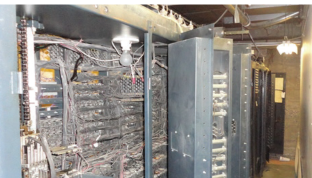
Modernized by Westinghouse in the 1960s with RSBL VV control
