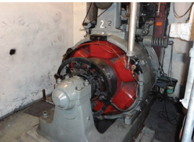
Early 1900s gearless basement traction elevators
