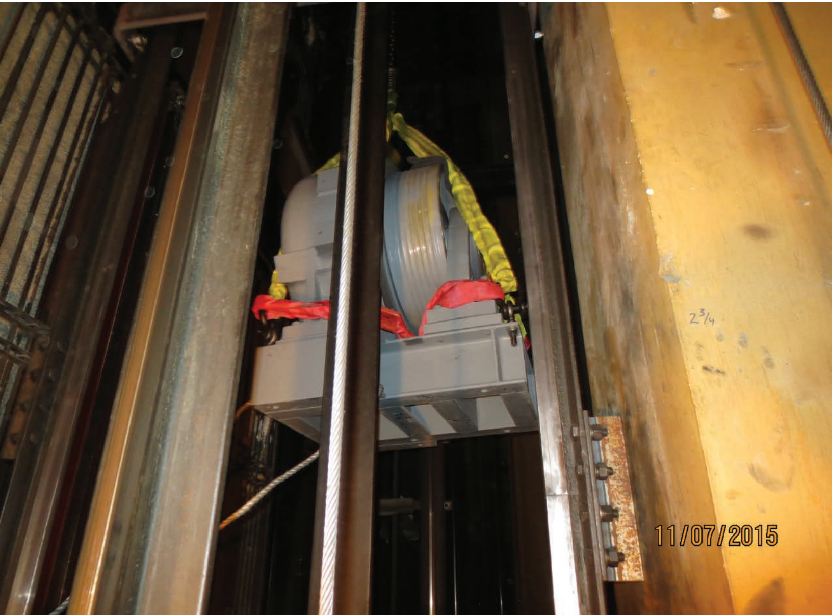
Hoisting up new equipment through elevator shaft. This was necessary because no crain can be used on this location on Market Street in San Francisco.
