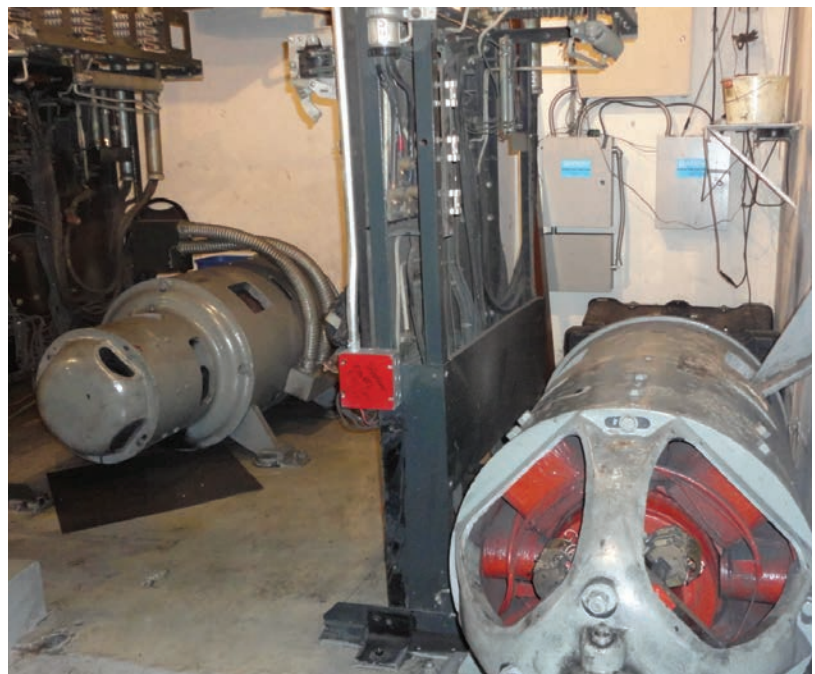
Existing motor drive technology was variable voltage control to a DC gearless hoistmotor – very common in the 1900s
