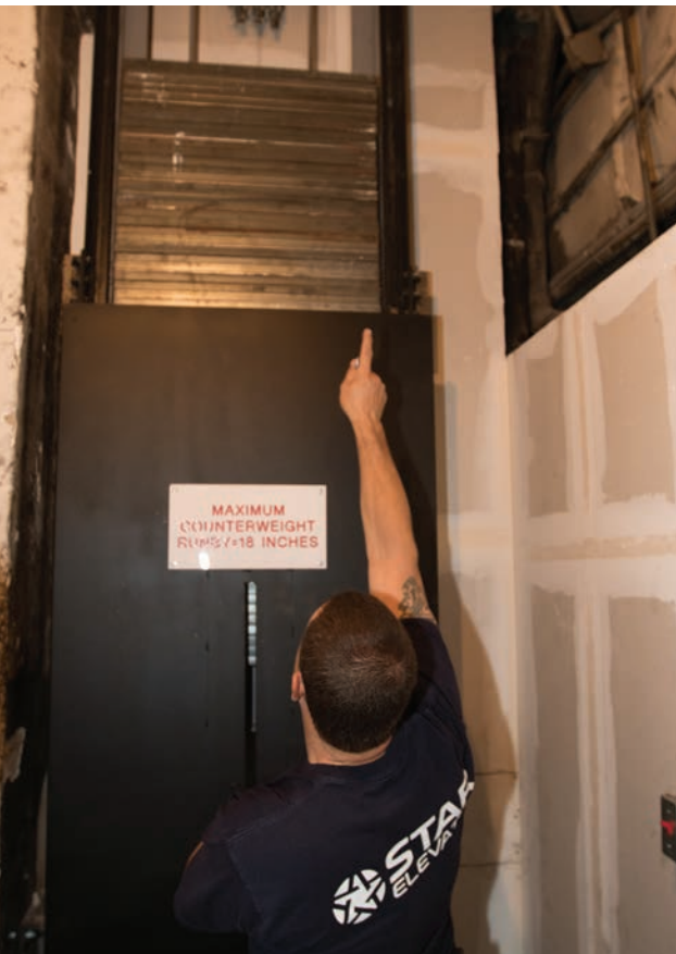
The distance between the counterweight rails was too small for the installation of new counterweights. So on each elevator, one counterweight rail stack had to be moved out over 10" to accommodate the new counterweight frame.
