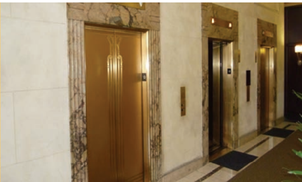
Three elevators, originally with manual car-switch operation had been updated to push button switches at some point.
